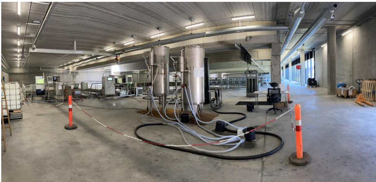
Figure 11. GAC pilot plant filters with samplings points at WWTP in Hillerød.
