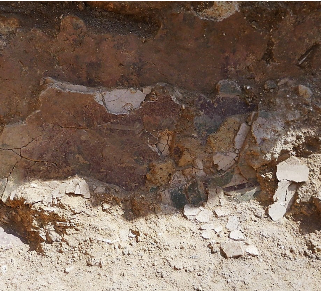
Photo from trench S, ev. J16-Sk-75, showing how the wall-paintings had fallen of the wall (© The Danish-German Jerash Northwest Quarter Project).
