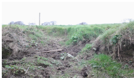
Figure 2. Poaching of channel bank.
